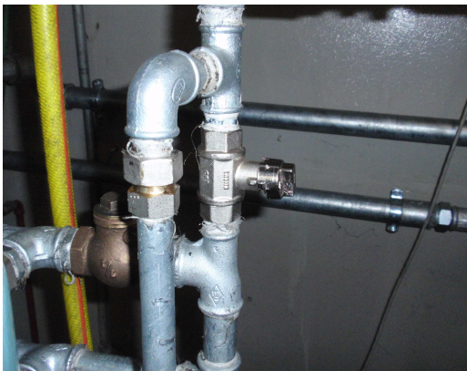
Alarm test valve "anti-tampering"
