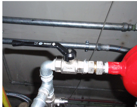
Alarm mute valve
